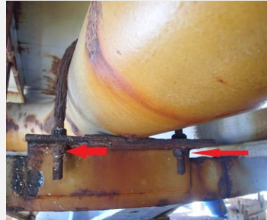
Stopped before detail design, issues with corrosion
